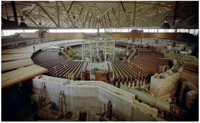
Overview of the Berkeley Bevatron during its construction in the early 1950s. One can just see the man on the left.
