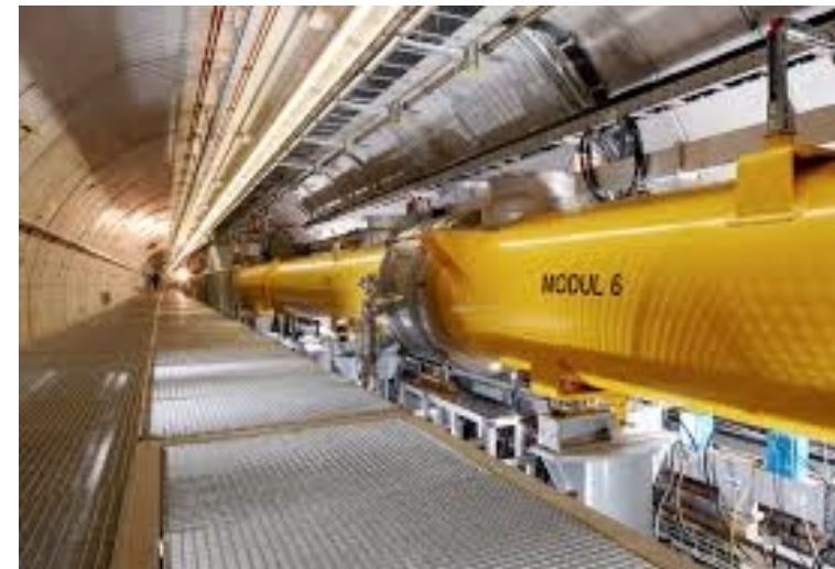
FLASH SC linac, at DESY, in Hamburg, Germany.
