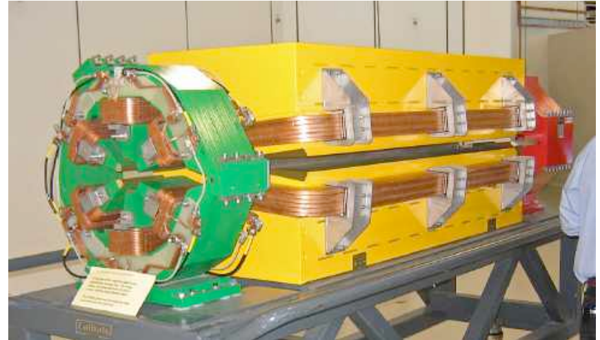
A magnet cell of an Australian light source: Green is a sextupole, yellow is a combined function dipole and red is a quadrupole
